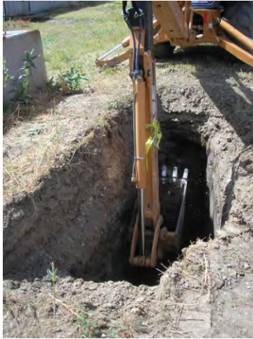
Sample collection from south wall. Flag tied at five feet above bucket.
